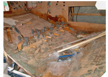
TOP: Clamps and poly around the glue area to prevent gluing the clamps to the stringers.
